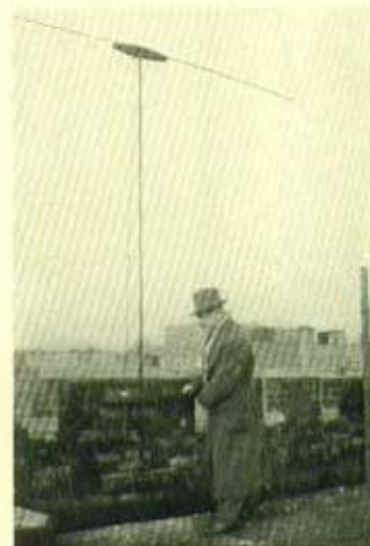
Fig. 3. A good antenna installation. Mounted in the clear and securely fastened by expansion bolts. Twisted-pair feeder is used
