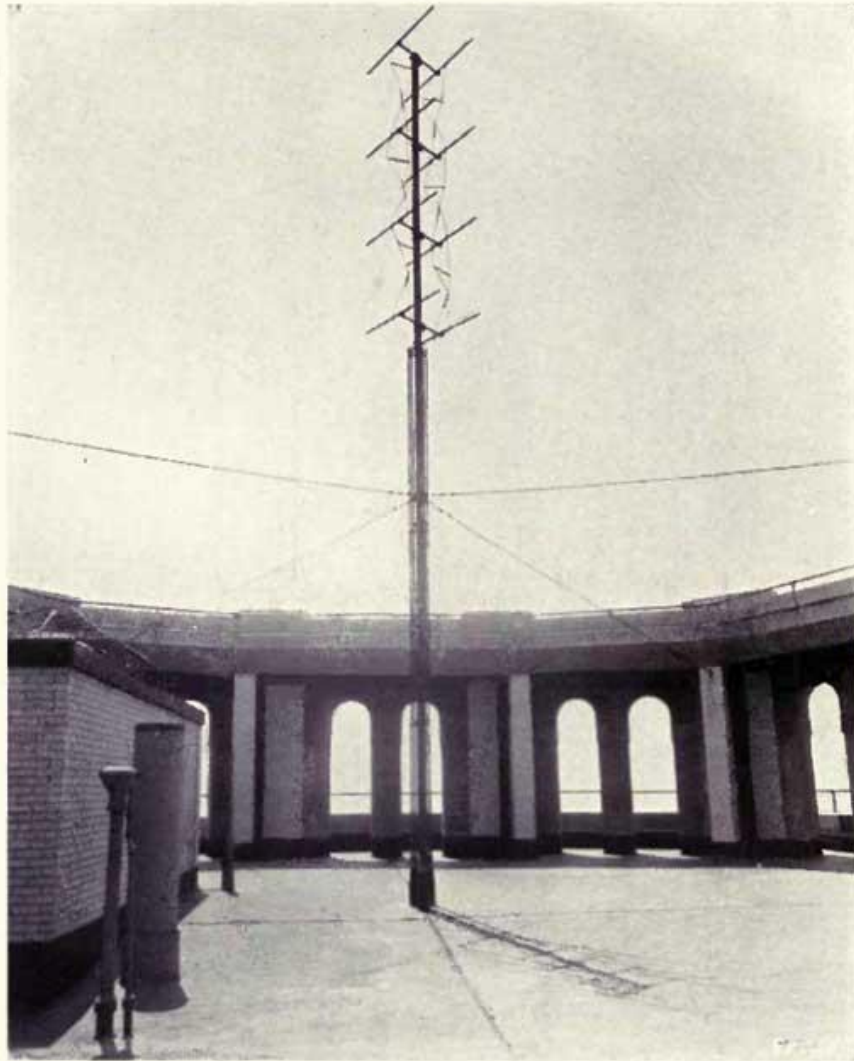
Fig. 80. Antenna Atop an Office Building in New York for Reception of Ultra-Short Waves, in the New York-Philadelphia Circuit of R.C.A.
