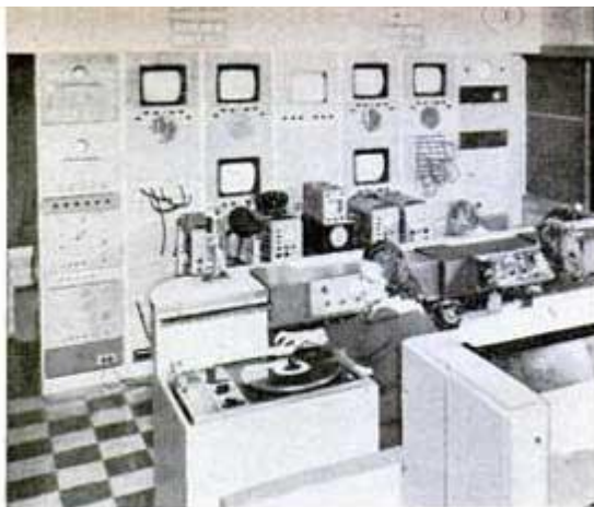
CONTROL ROOM where engineers, technical directors, and producers check details of program.
